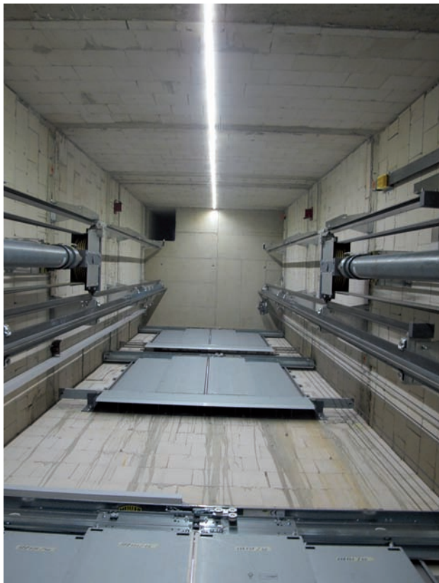
Mounting example: Goods lift, load capacity 1.6 t with a shaft surface of 6.4m 2
